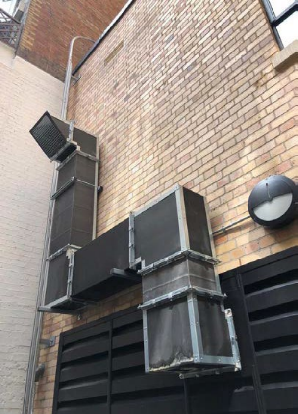
Smoke extract duct
