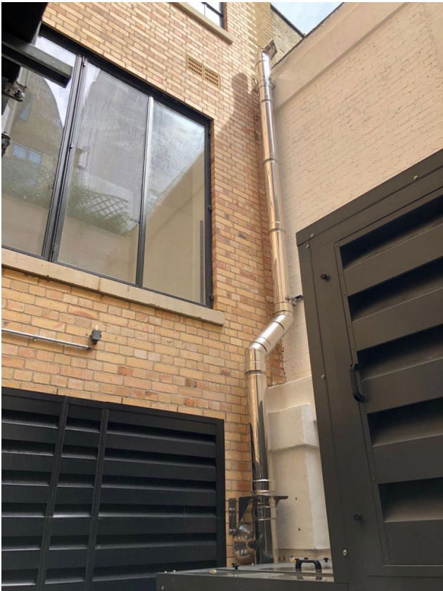
Generator exhaust flue
